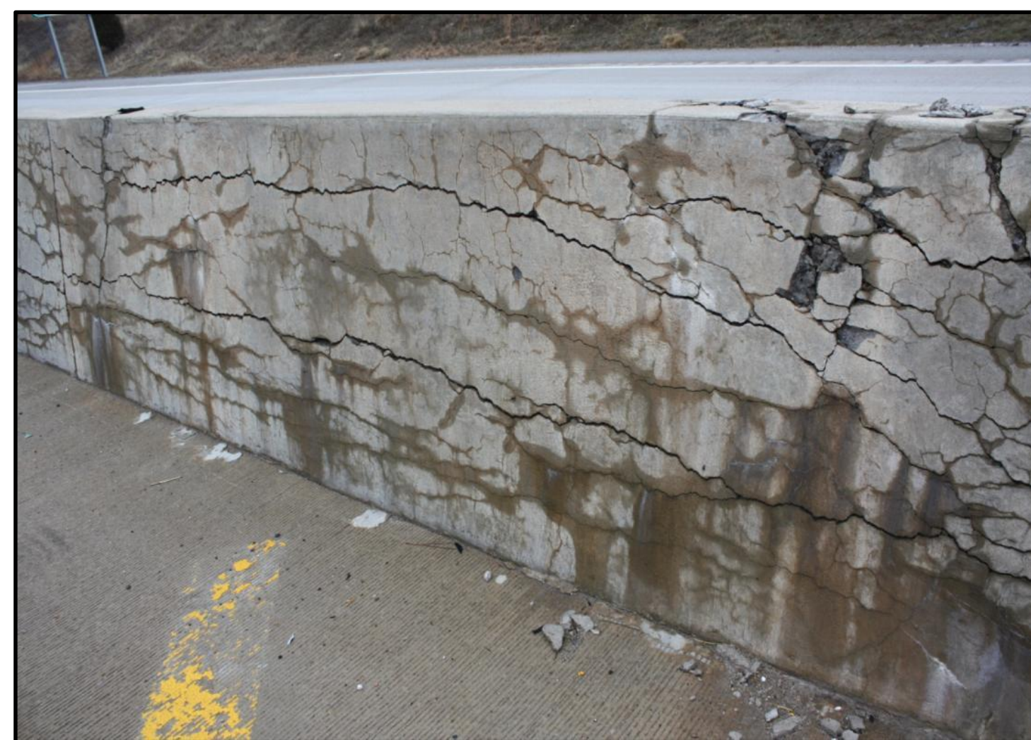
Barrier wall exhibiting ASR deterioration
