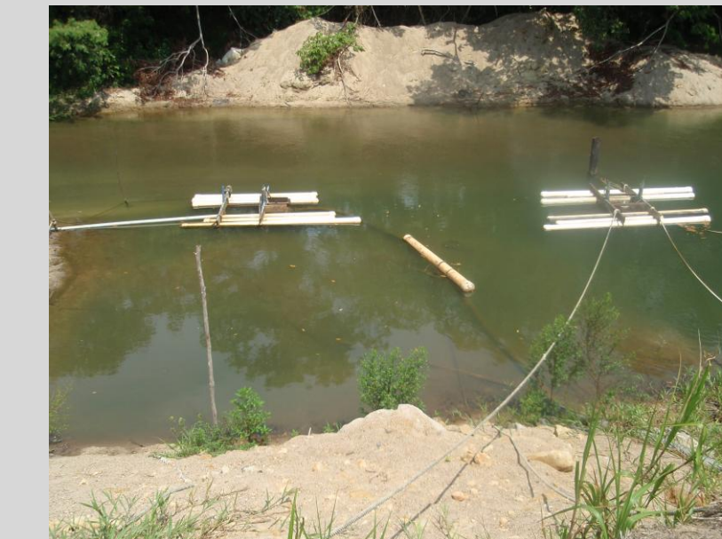
Pumping station at Dangriga's water facility in North Stann Creek
